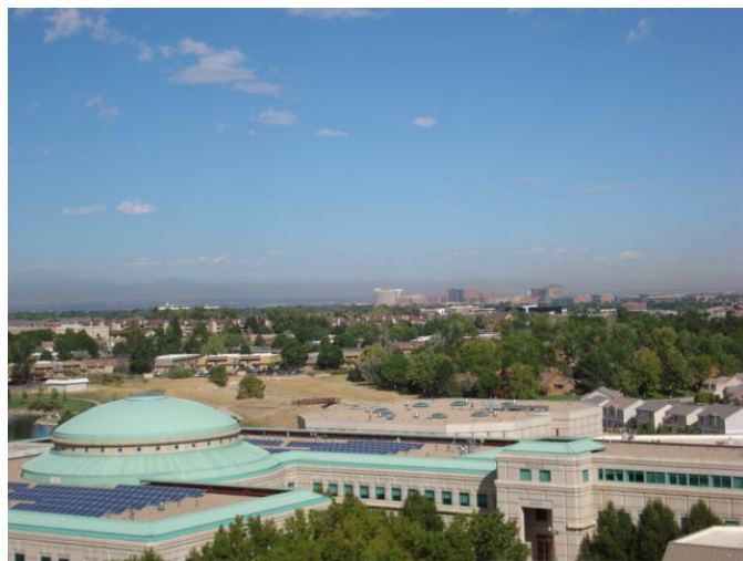
A 100 kw solar PV installation on Aurora's municipal court building is financed through a power purchase agreement.
