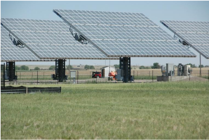
Solar panels at Solar TAC on the Aurora Campus for Renewable Energy.
